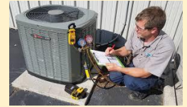
HVAC Heating & Air
